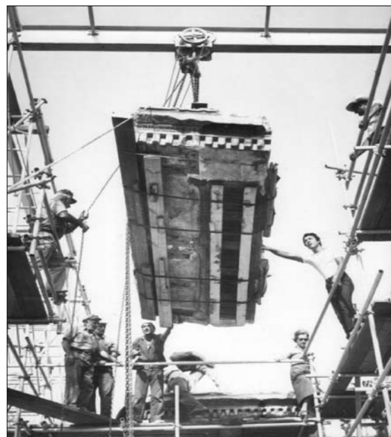
Transportation of the slab of the roof of the porch of the Karyatids (7 tons)
