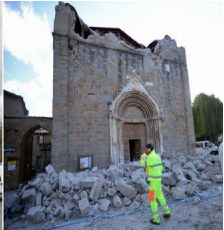
After the earthquake
